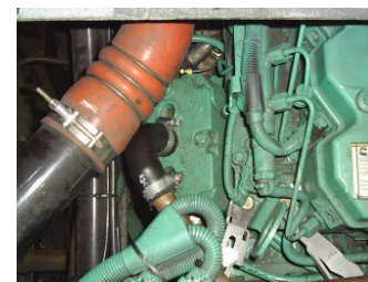
Check there is no damage or crushing of the compressor inlet pipe
